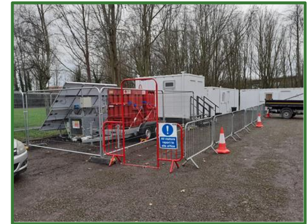
Figure 2: One of the Hydrogen Cells used to power the site.
