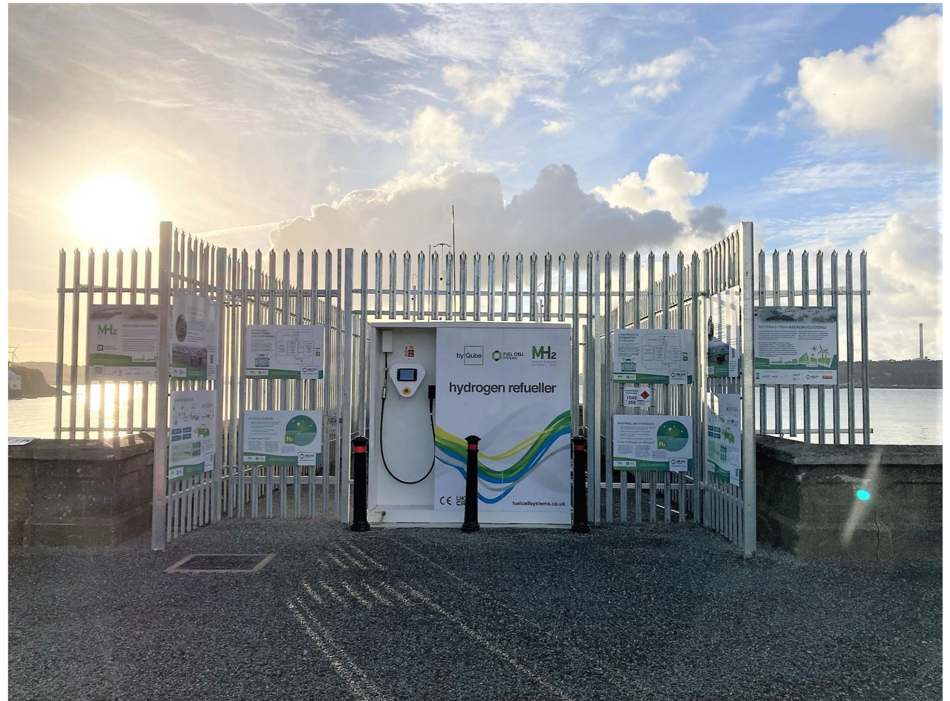
Figure 15: MH:EK hydrogen refueller demonstrator
