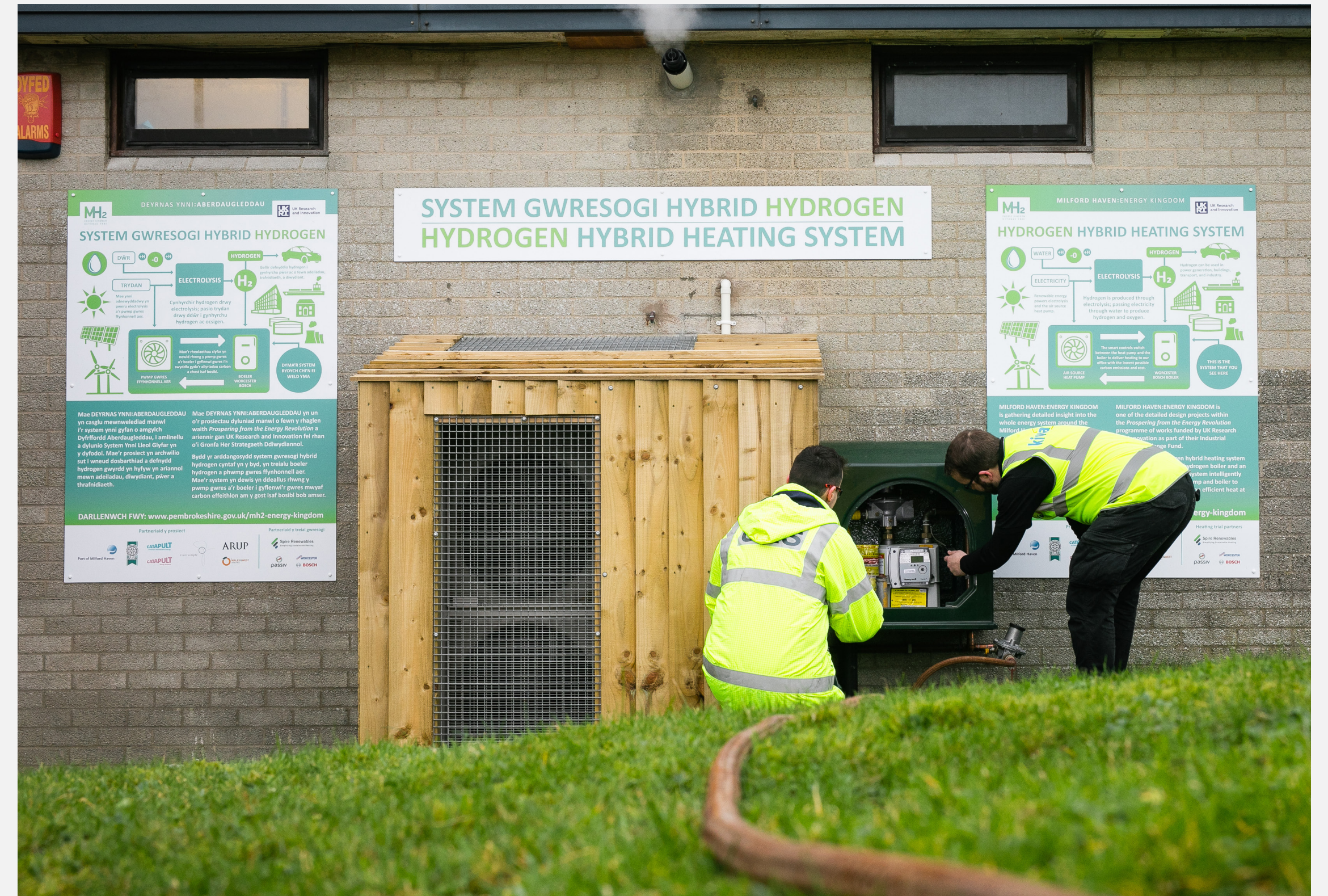
Figure 26 Hybrid heating system demonstration © Port of Milford Haven
